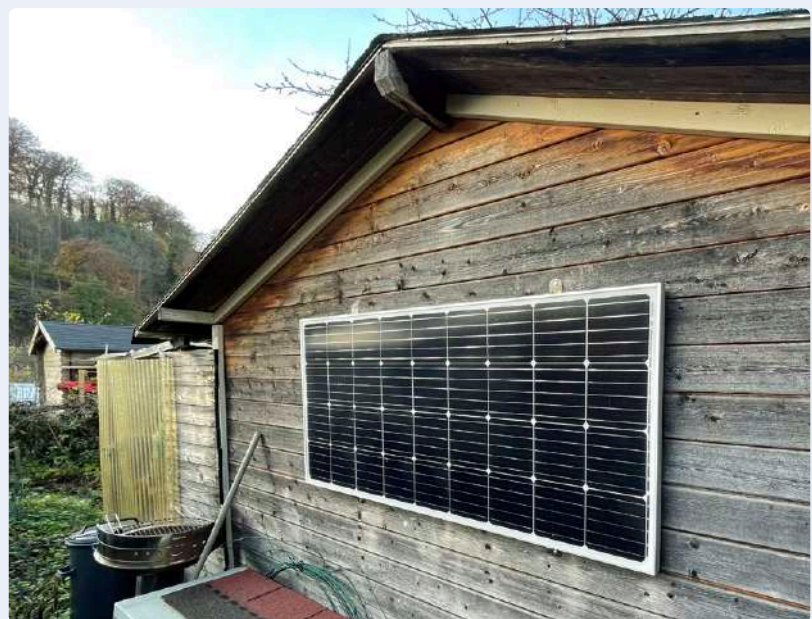
Figure 2: The 12 V solar panel mounted vertically on the wall of Klaus' shed. It has an output rating of 180 Wp.
