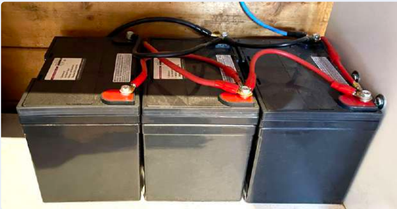
Figure 3: Three 12 V lead gel batteries, each rated at 36 Ah, are wired in parallel to act as energy storage in Klaus' shed.
