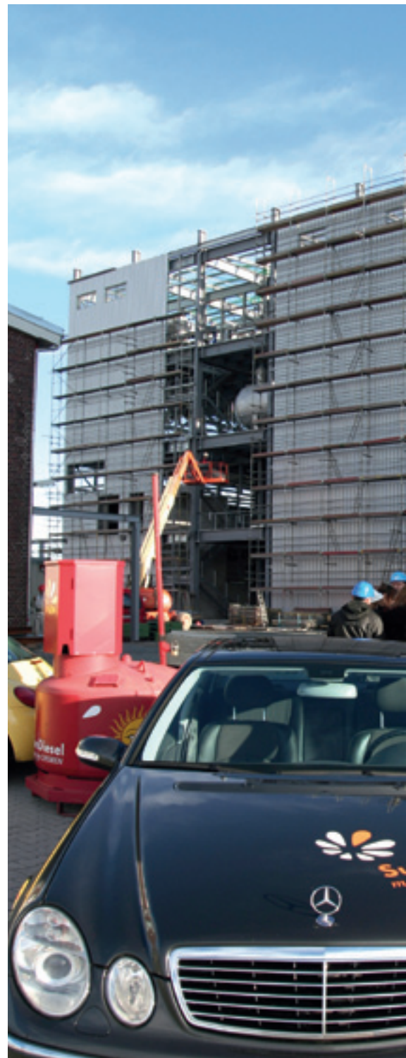
The Choren Company is building the world's first commercial plant for the production of Biomass-To-Liquid (BTL) fuels in Freiberg. This so-called Beta plant will go into operation in the first half of 2008. Photo: Stefan Schroeter.
