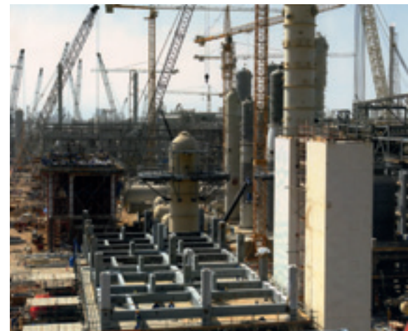
The first of Qatar's six 4.8 mtpa mega-trains is under construction. Each of these huge installations is about one kilometre long.
