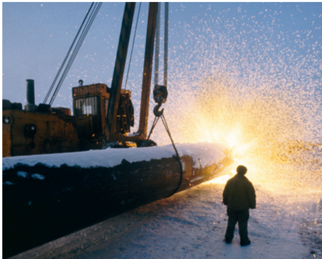
A rotating welder is used during construction of the Trans-Siberian gas pipeline. Photo: Fabian Cevallos, Corbis
