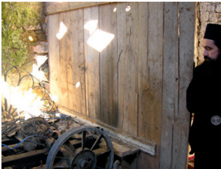
Father Gavriilo shows the broken pump of the watermill. Photo: Anke Truijen
