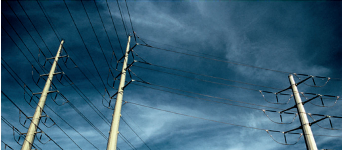
The fact that Europe is still using an outdated electricity grid, while the energy market is on the threshold of an enormous turn-about, worries the European Commission. Photo: image100/Corbis
