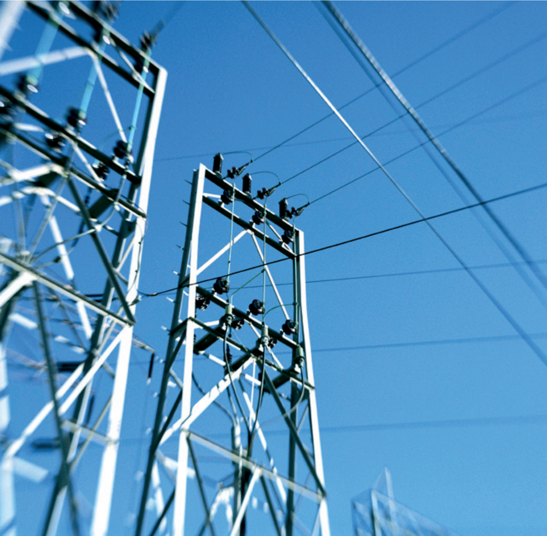
High voltage power lines and transmission tower. Photo: Stewart Tilger/Corbis
