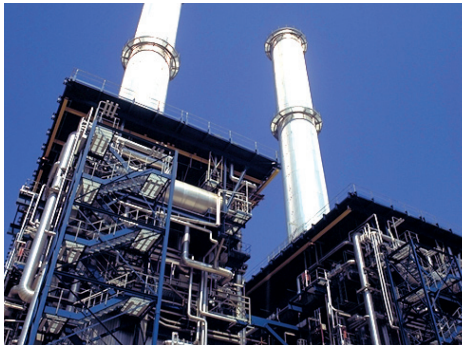
DEI gas fired power station. Photo: Public Power Corporation S.A.
