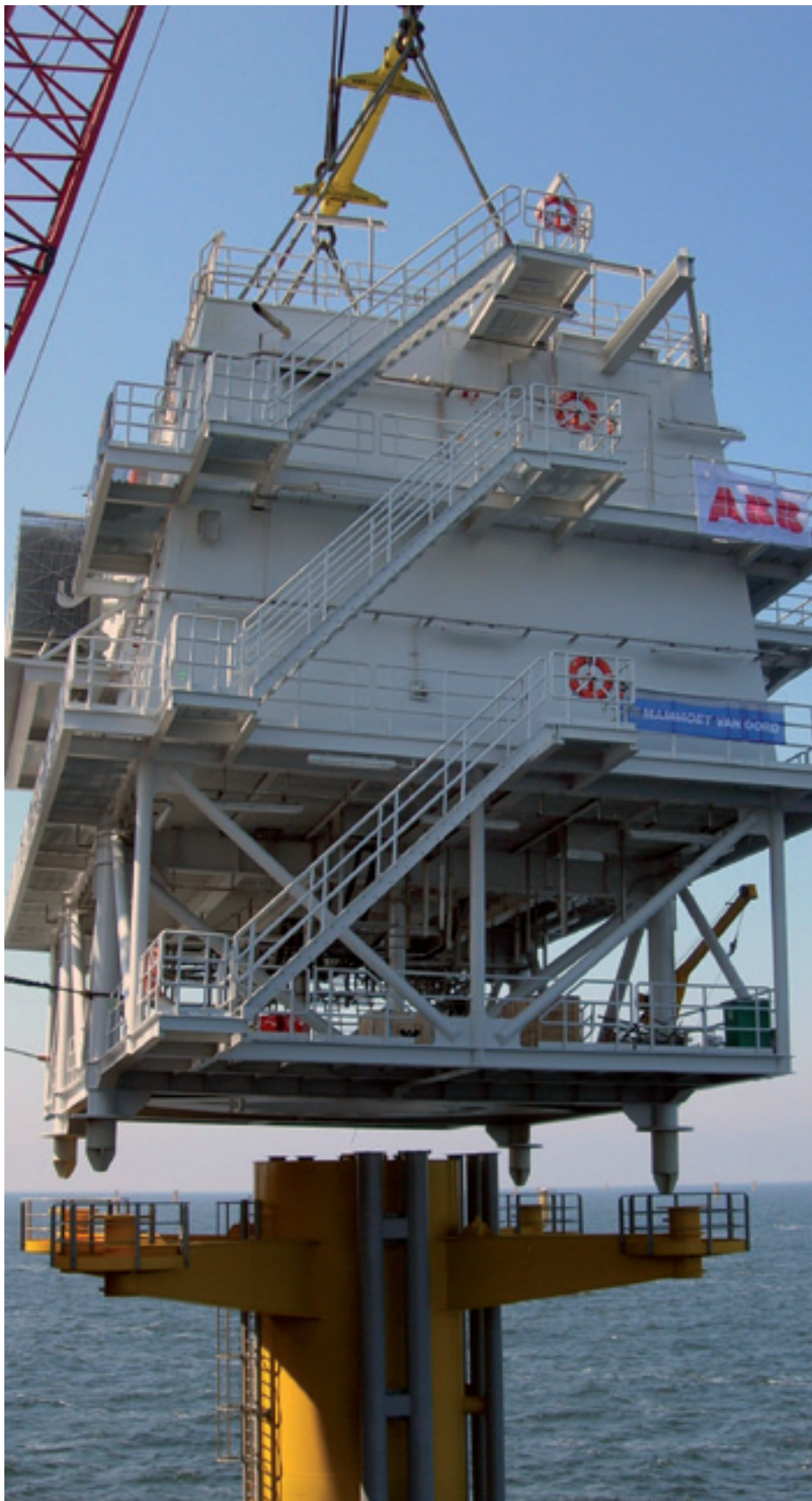
The installation of a transformer station weighing 650 tonnes. Photo: Econcern
