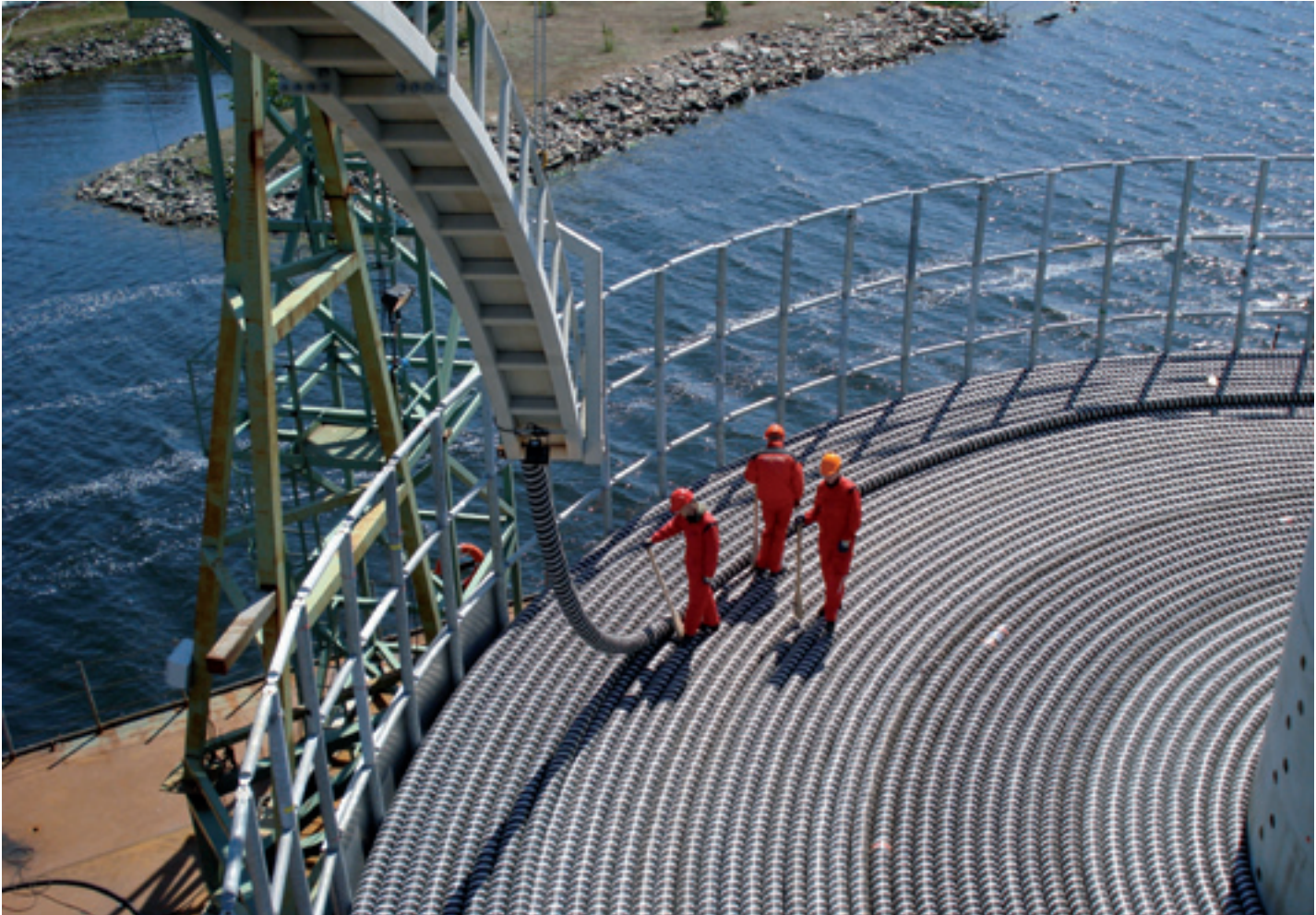
A 23 kilometre cable is transported on a special winch. This picture shows a spare section of the cable, to be used in the case of a breach, which is taken off the winch to be transported to a storage facility. Photo: Econcert
