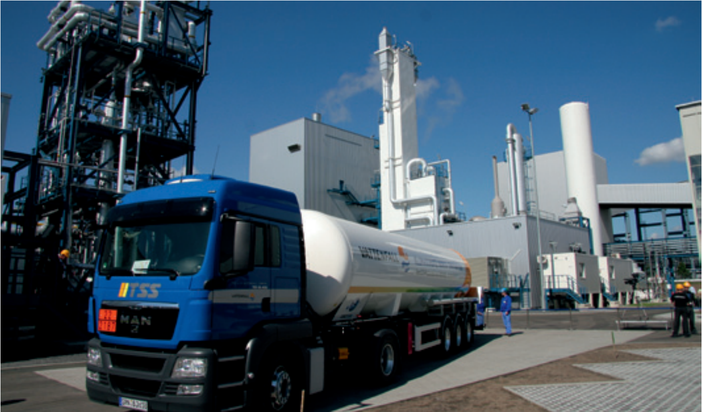
Oxyfuel carbon capture plant at Schwarze Pumpe Photo: Stefan Schroeter
