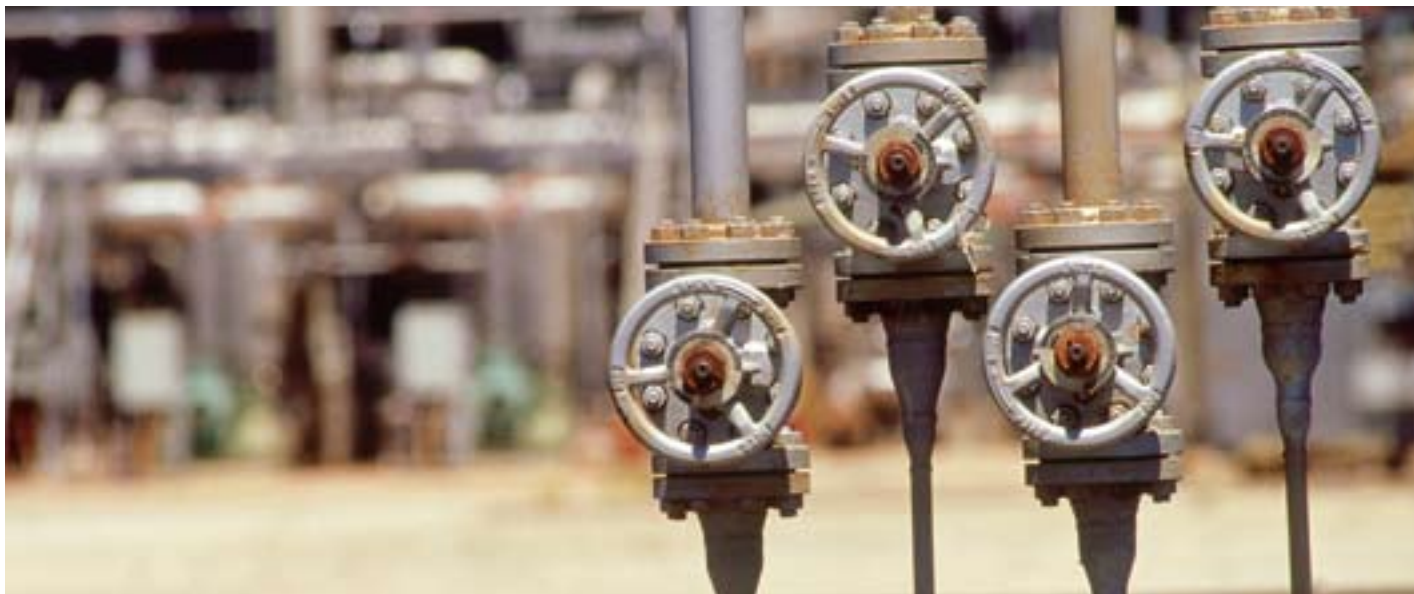
Set of valves at liquefied natural gas facility. Photo: Photolibary/Hollandse Hoogte
