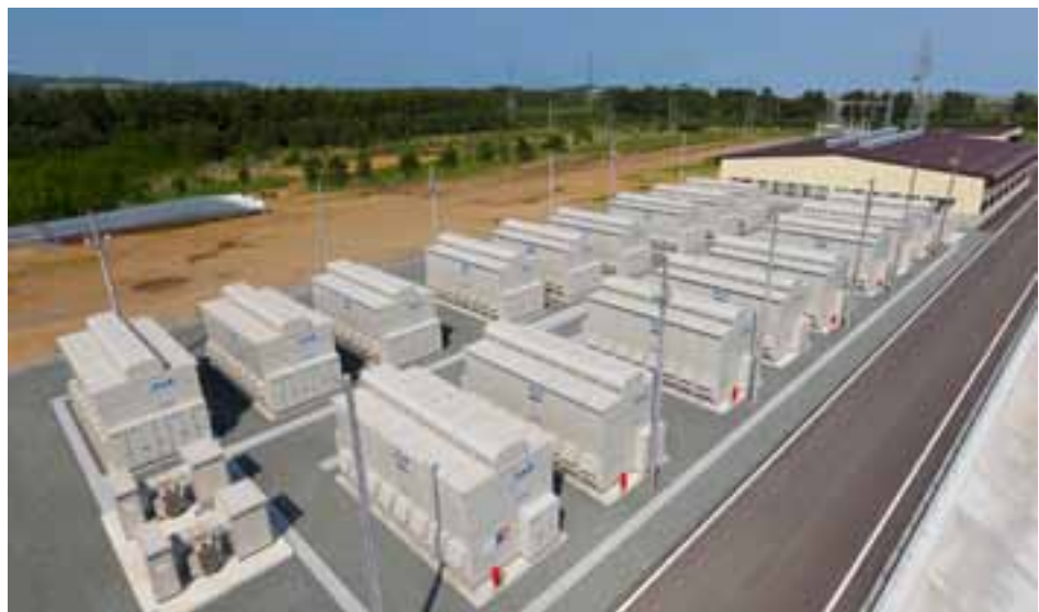
34 MW Sodium Sulphur Battery in Futumata, Japan. Photo: NGK
