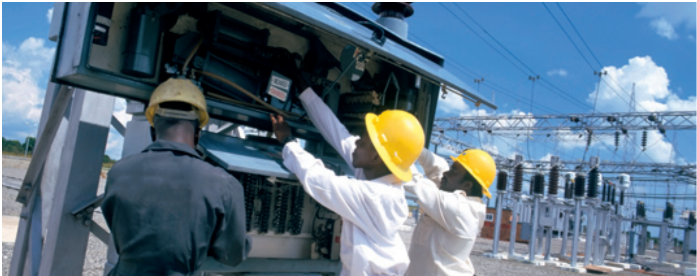
Electricity Substation, Zambia. Photo: Construction Photography/Corbis
