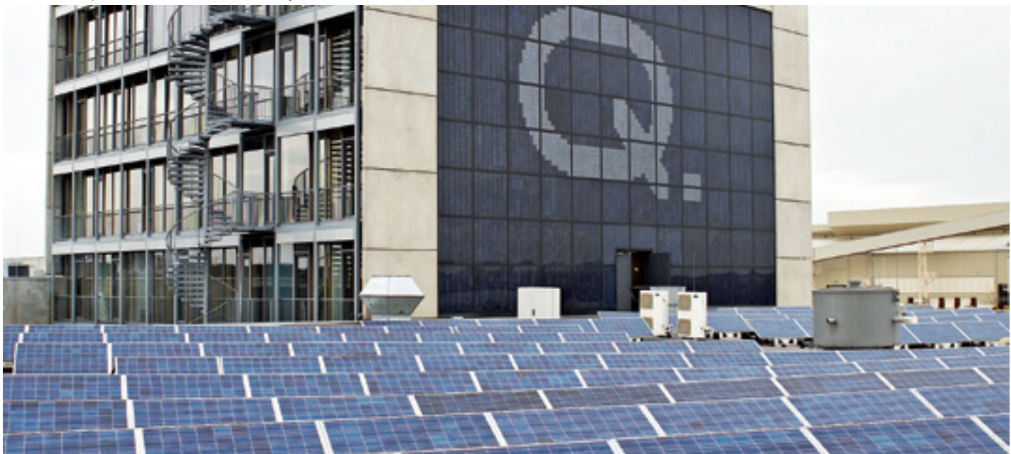
On the rooftop of Q-Cells at Thalheim, Germany. Photo: Kai Senf
