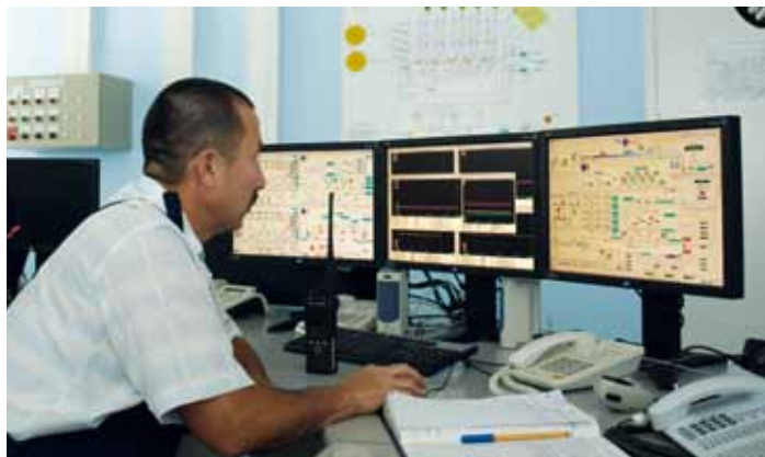
Control centre of CPC pumping station in Atyrau. Photo: Rudolf ten Hoedt
